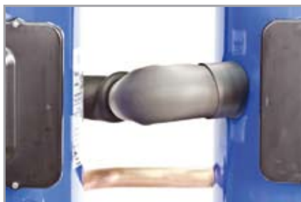
Suction line insulation
